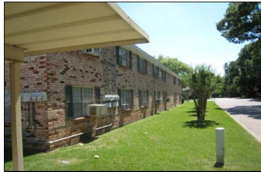
Individual Heating/AC Units
